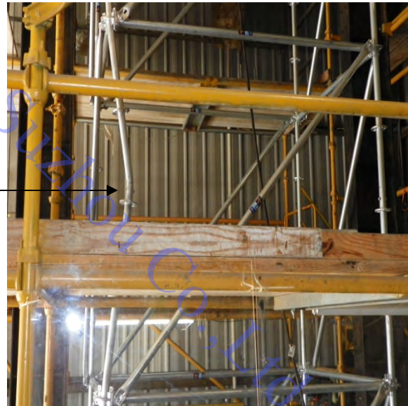
Typical deflection of leg at failure
